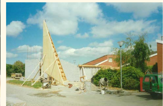
Construction of the MacDonnell Chapel at the Horowhenua Village, funded by a donation from resident Mrs Phyllis MacDonnell
